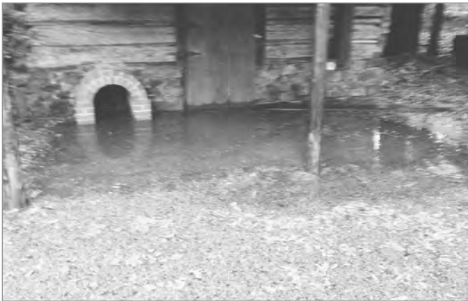
Standing water blocks entrance to Tobacco Barn.
