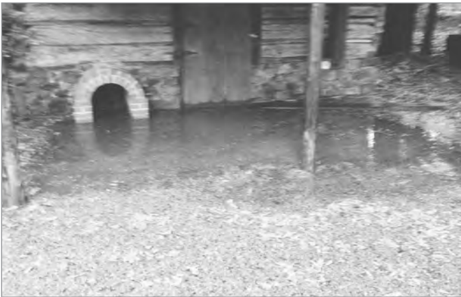
Standing water blocks entrance to Tobacco Barn.
