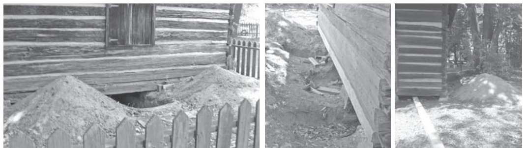
Below: Photos of the current repair project which involves digging underneath the cabin.
