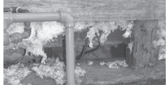
The underbelly of the Shaw House needed extensive work to strengthen the foundation by replacing rotten wood and re-doing some electrical work to bring it to code.
